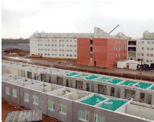
Right and below: PCE's structural solution is based on a fast-track formula for precast crosswall construction.
